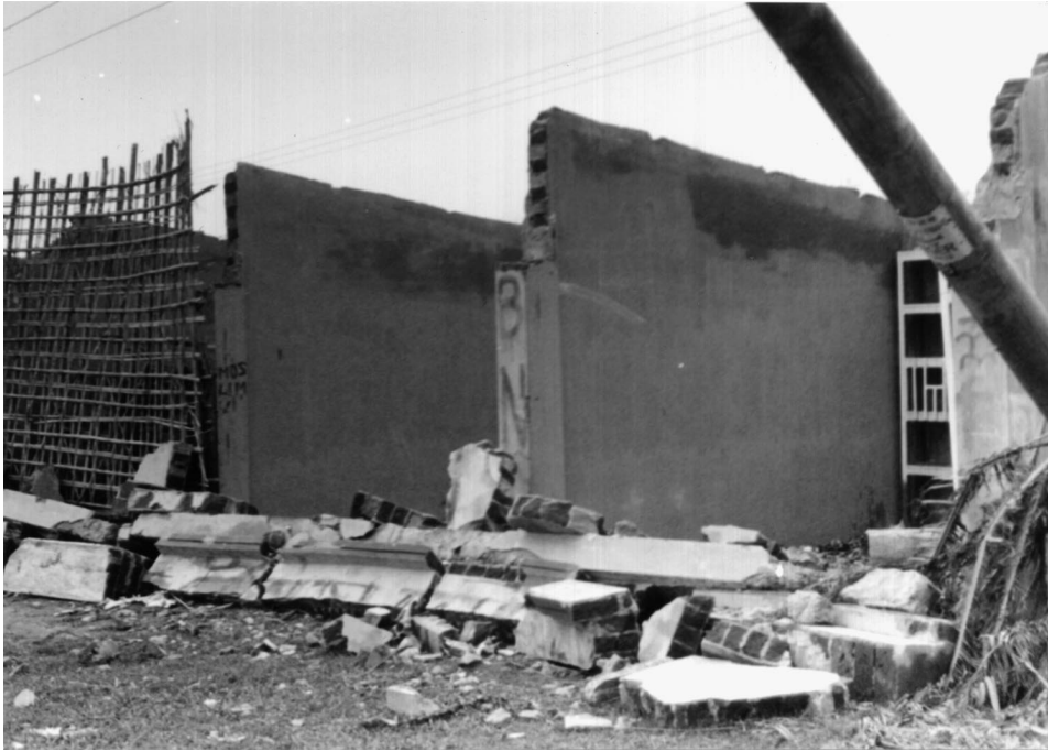
Figure 4. A retail shopping area in Bandar thana where cyclonic winds destroyed roofs and walls. Masonry buildings often cannot withstand the high-velocity winds. Although material losses due to cyclones are high in urban areas, the loss of human lives is comparatively lower here than in rural and island communities.
