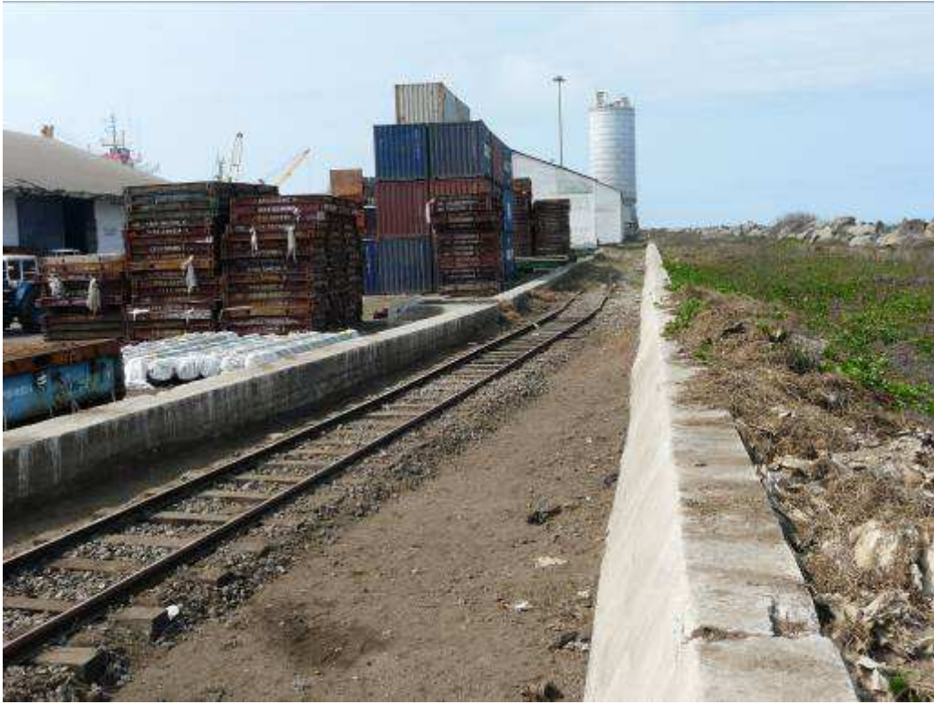
7) State of the rail road at the port area
