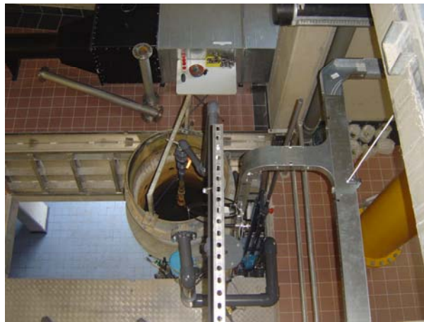
Figure 3.1: Pilot plant built inside Harderbroek
