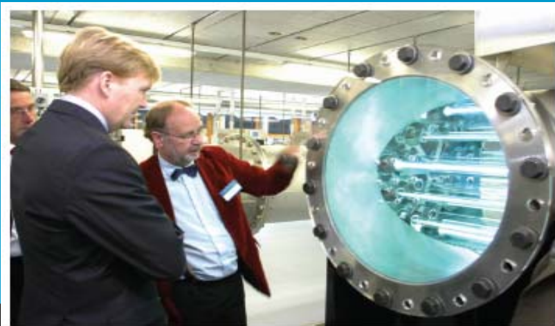
UV for disinfection at Andijk (PWN 2005)
