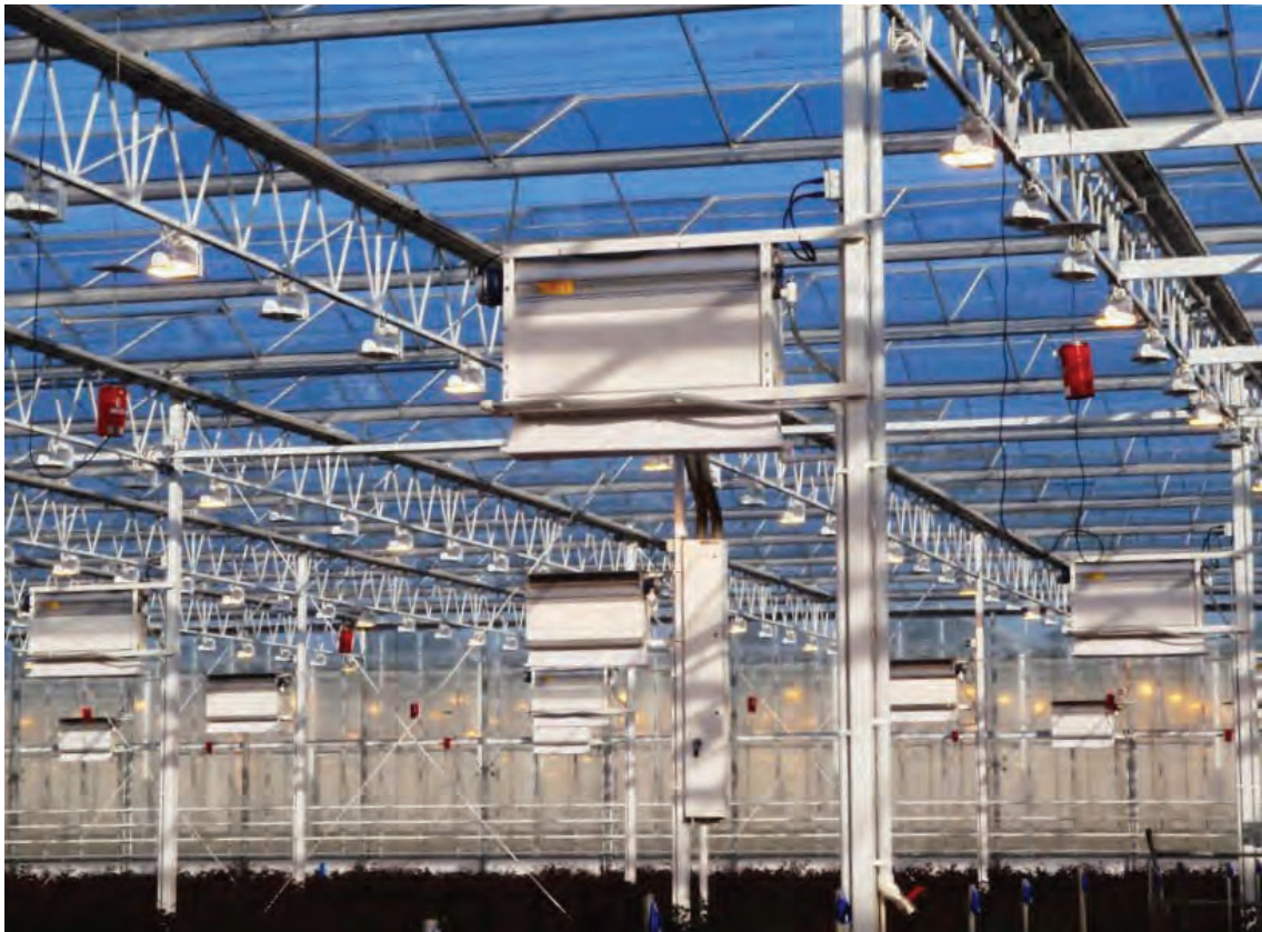
Fig. 04.27: Fiwihex hanging in a rose greenhouse for heating and cooling
