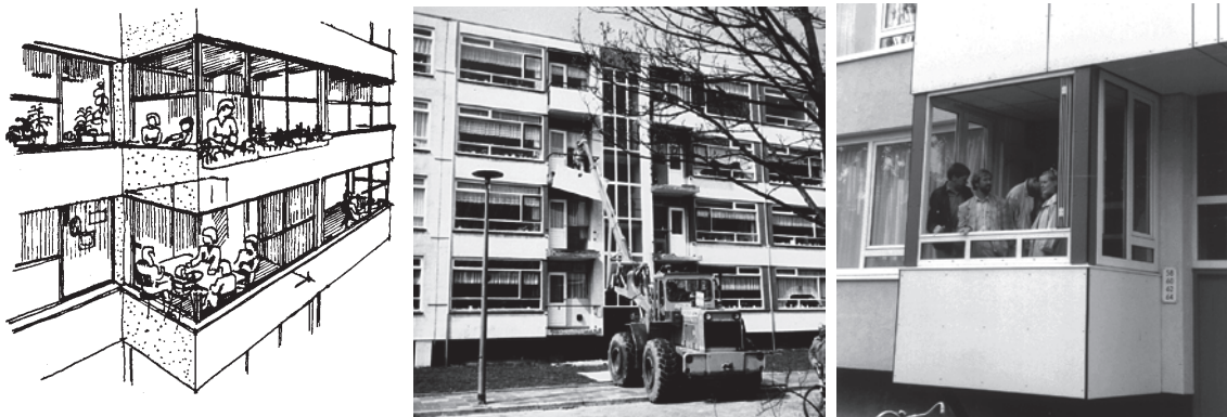
Fig. 04.20: Impression of the new balcony, removal of the balconies and a new one in place
