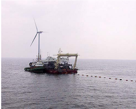
Specialised installation with existing equipment
