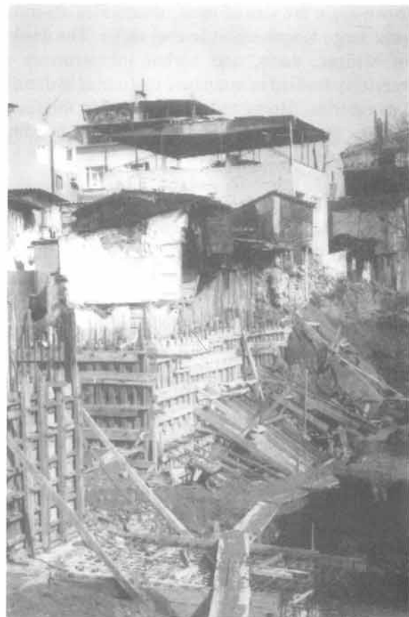
Figure 16-2: Excavation at construction site with scaffolding of the walls in the foundation works.
