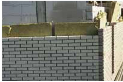
Fig. 2.17: Careful implementation reduces energy loss. The picture clearly shows that the insulation does not fit together, causing serious thermal leakage
