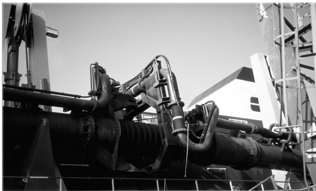
Figure 2-78 Jet pipeline passing the universal joint
