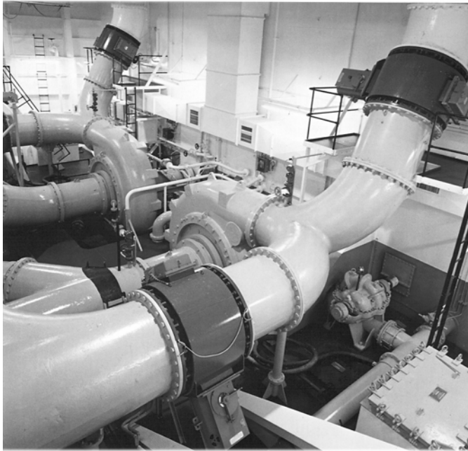
Figure 2-30 Pump room with 2 pumps
