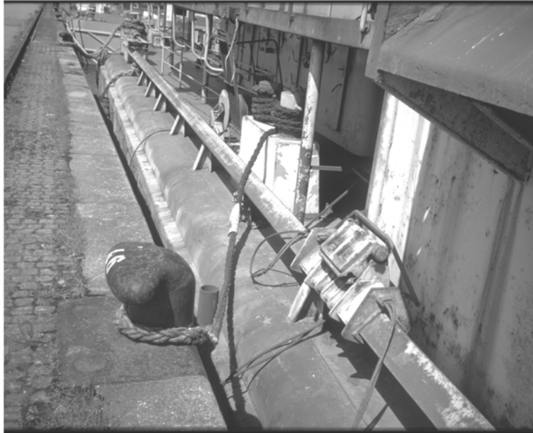
Figure 5-13 Sliding part of the Barge Hauling installation
