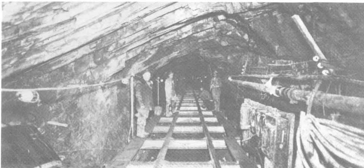
Figure 1-9a: The structure of the rock formations greatly affects the strategy and final shape of tunnel construction. View inside the City Tunnel, Boston, during its construction.
