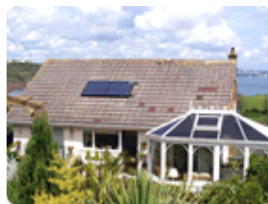
Figure 2: Solar panel installed on a rooftop (source : www.solartwin.com ).
