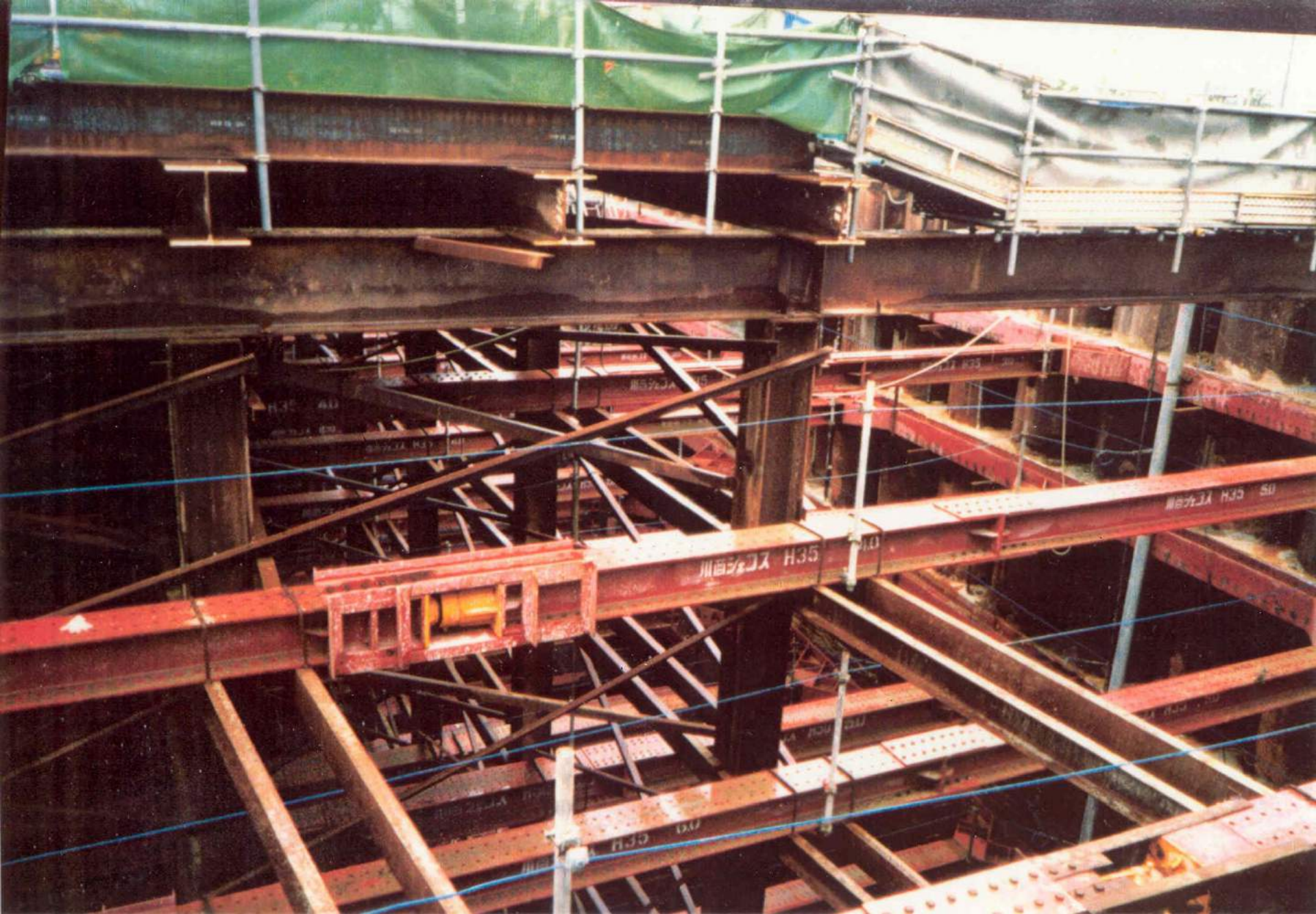
A lot of struts can be used to keep the building pit stable (note the jack)
