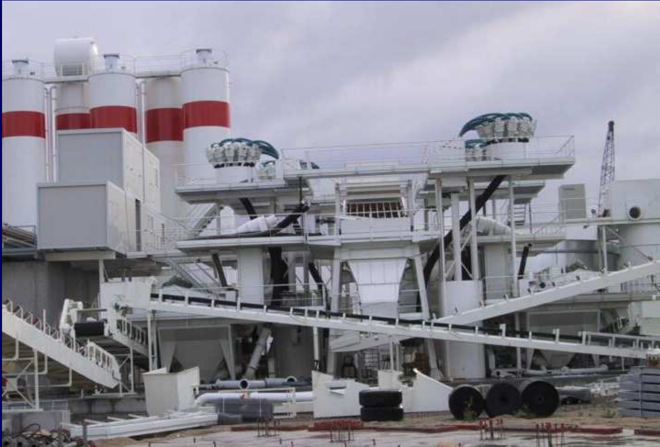
Separation plant Groene Hart, 2500m 3 /hr supplied by MS in 1998
