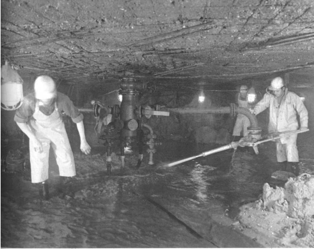
Figure 5.13: Personnel working in space beneath the caisson of the East-line in Amsterdam
