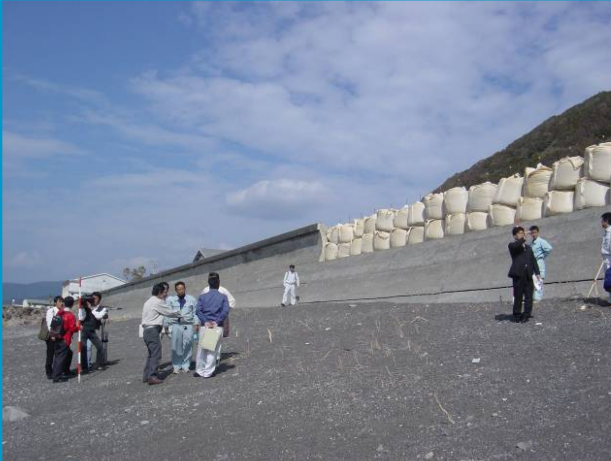
Damage due to typhoon Tokage (Oct 2004) Muroto Kochi, Japan
