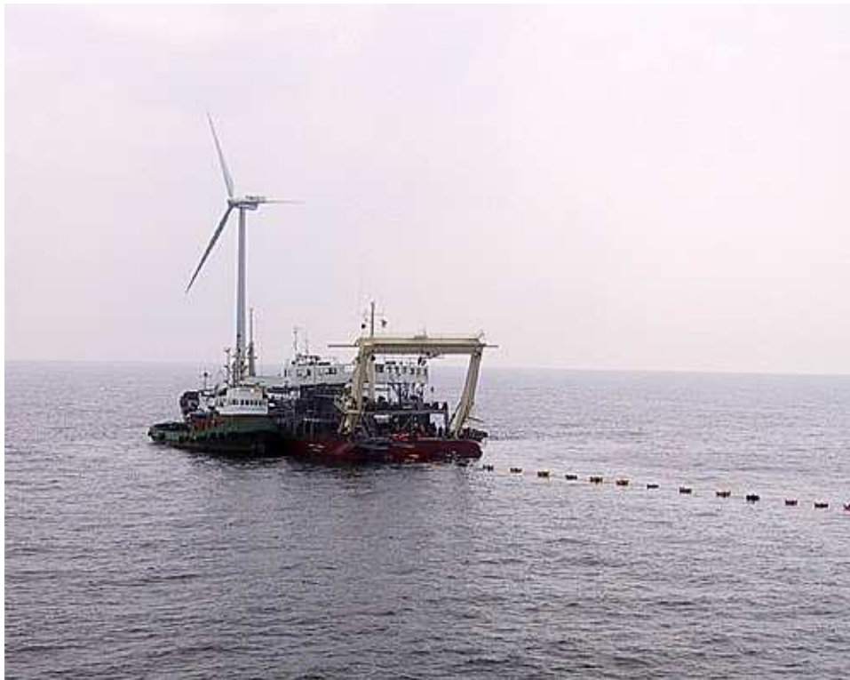
Specialised installation equipment (existing)
