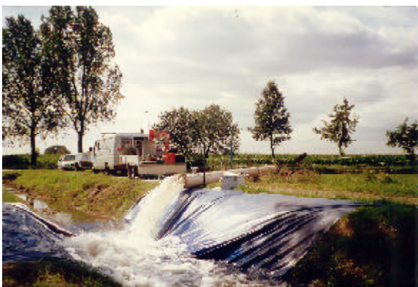
Fig. 7.10 - Dedicated flushing point
