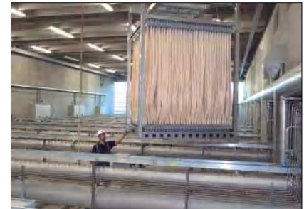
Figure 2.9 Low-pressure immersed UF
